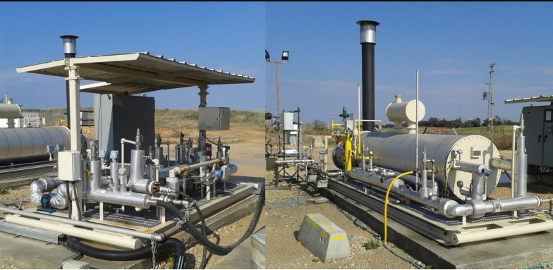
The Heletz deep-well CO 2 injection facility (EWRE, Israel)
